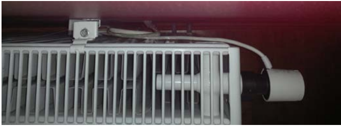
Fig. 3. Thermal driver allowing to control the valve via RPi computer.
